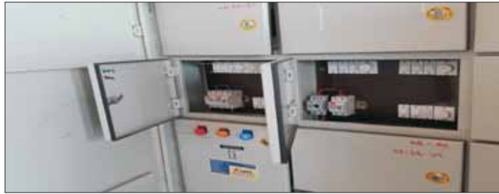
Centralized controlling unit for lights, fans etc. inside the cells.
